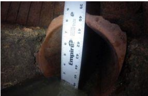
Monitored Pipe Size
