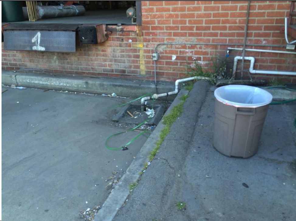
Photo #7 View of storm drain and sump located along the southwestern exterior of the building.
