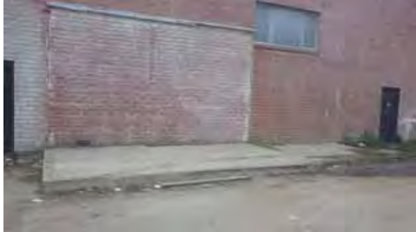
View of area of raised cement adjacent to west exterior of building
