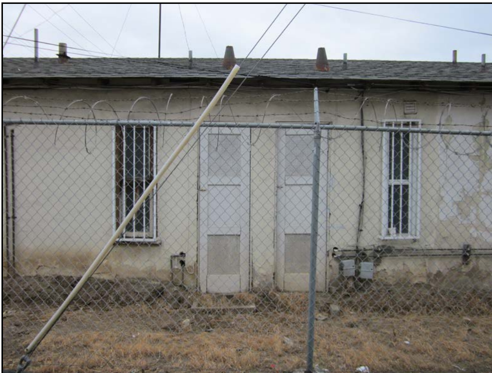
Access doors to water boilers, north elevation
