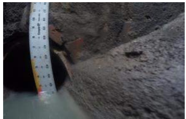
Monitored Pipe Size
