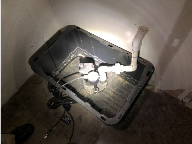
View of a pump in the room
