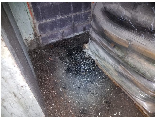
View of the oil stains around the pallets at the southeastern corner of the building
