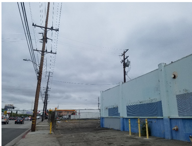
View of a pole-mounted transformer
