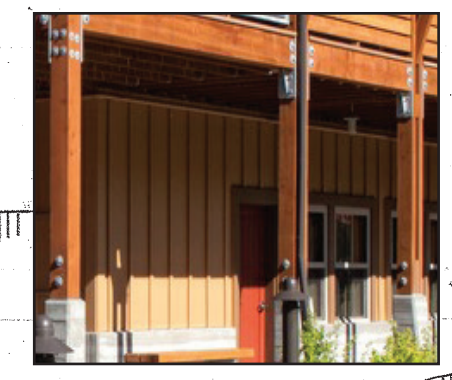
Stained T-111 siding
