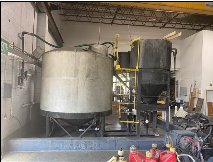
9. View of water treatment system
