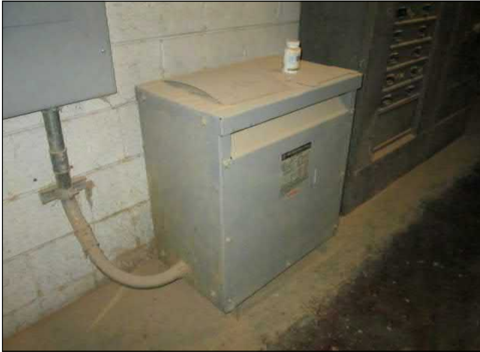
Photo 15: One of two dry-type transformers within the industrial structure.
