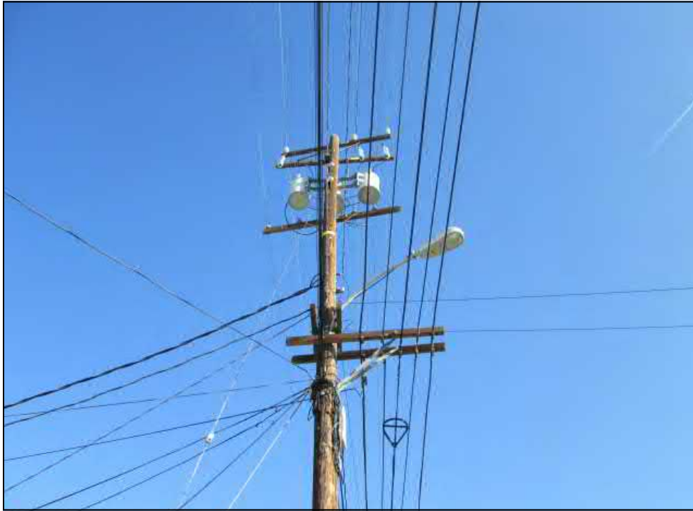
Photo 3: View of the pole-mounted transformers in the northeast corner of the subject property.
