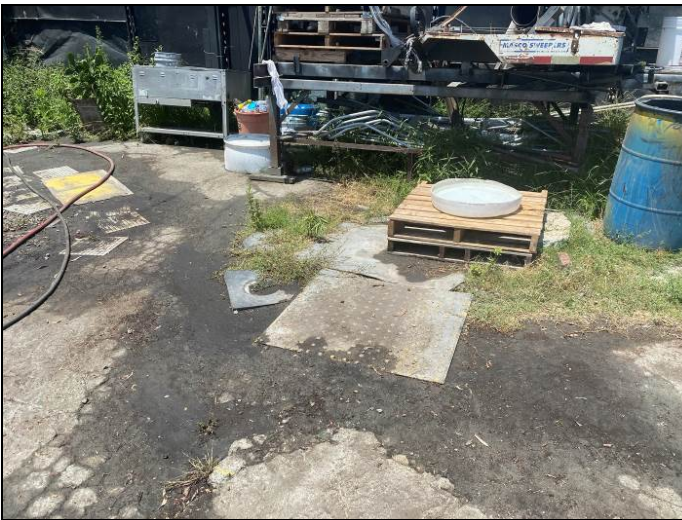
15. View of sludge staining in southwest corner
