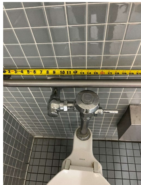
Rear Grab Bar location
