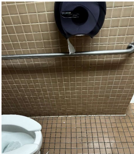
Men's Toilet Paper Dispenser (wrong location)
