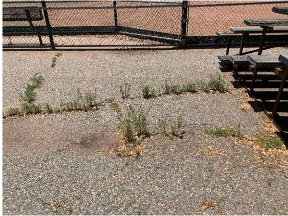
Typical asphalt condition at ballfield
