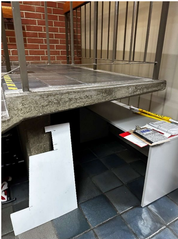
Non-compliant clearance under stair landing
