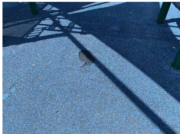
Rubberized Surface Damage
