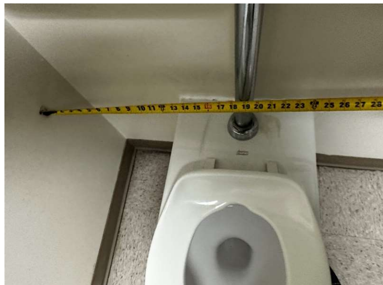
Toilet centered too far from side wall
