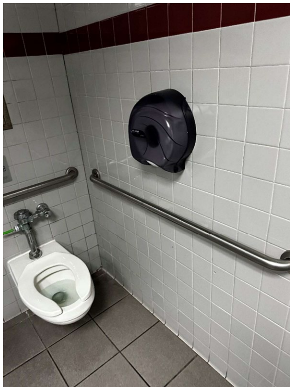
Toilet paper dispenser incorrectly located
