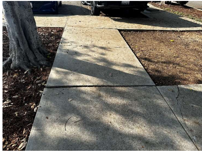
Heaving Concrete Walkway
