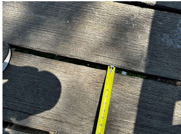
Typical Bridge Plank Gaps
