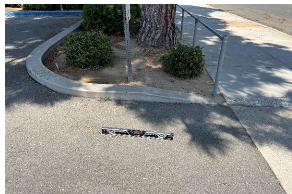
Non-compliant Path of Travel from Parking Lot
