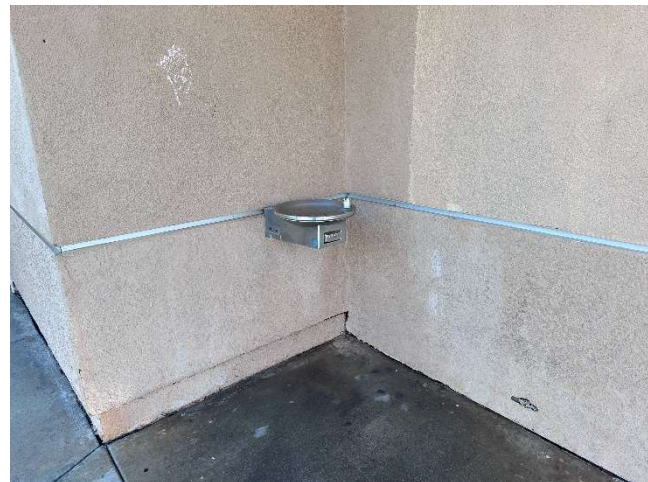
Non-compliant drinking fountain
