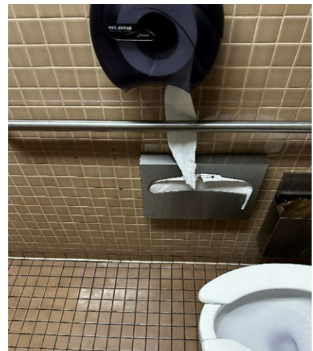
Women's Toilet Paper Dispenser (wrong location)
