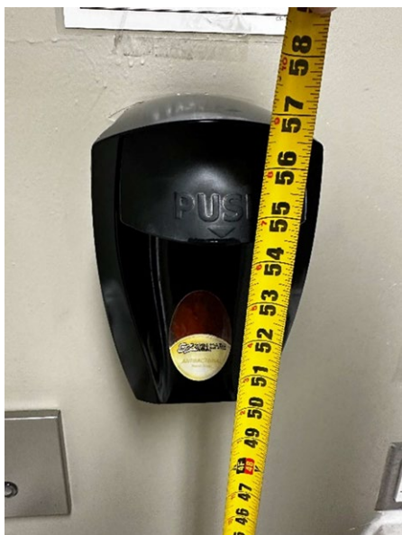
Men's non-compliant dispenser height
