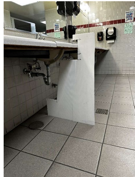
Missing insulation on pipes
