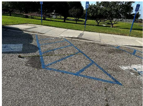
Typical Non-compliant Curb Ramps
