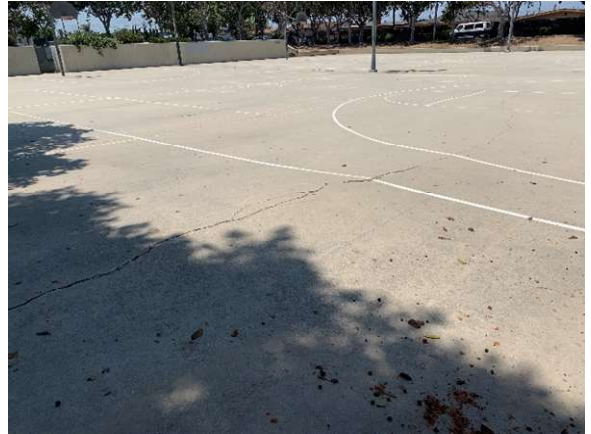
Cracked Basketball Courts
