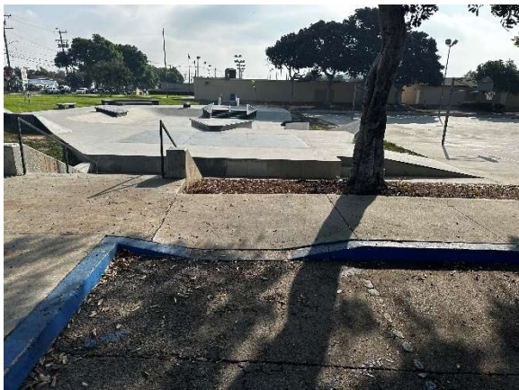
Non-compliant Curb Ramp 1
