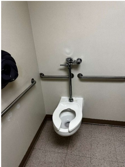
Non-Compliant Rear Grab Bar
