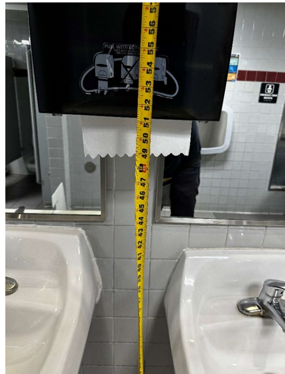
Dispenser height too high
