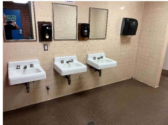
Men's Restroom Lavatories
