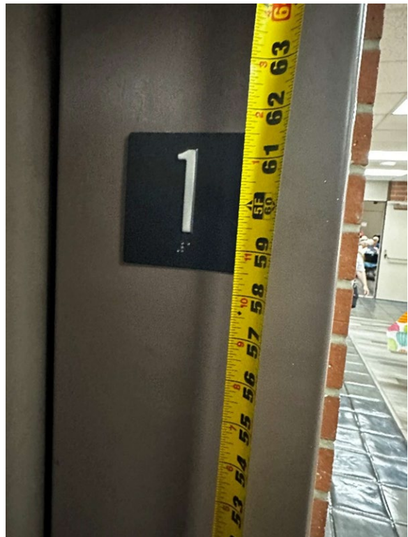
Incorrect Jamb Signage at First Floor Landing
