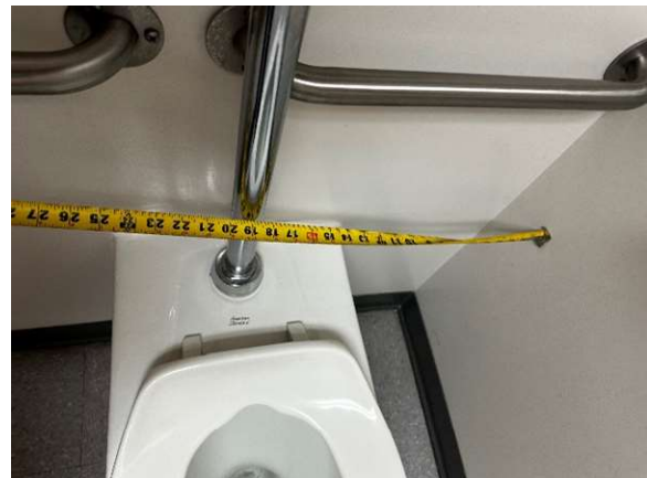
Toilet centered too far from side wall
