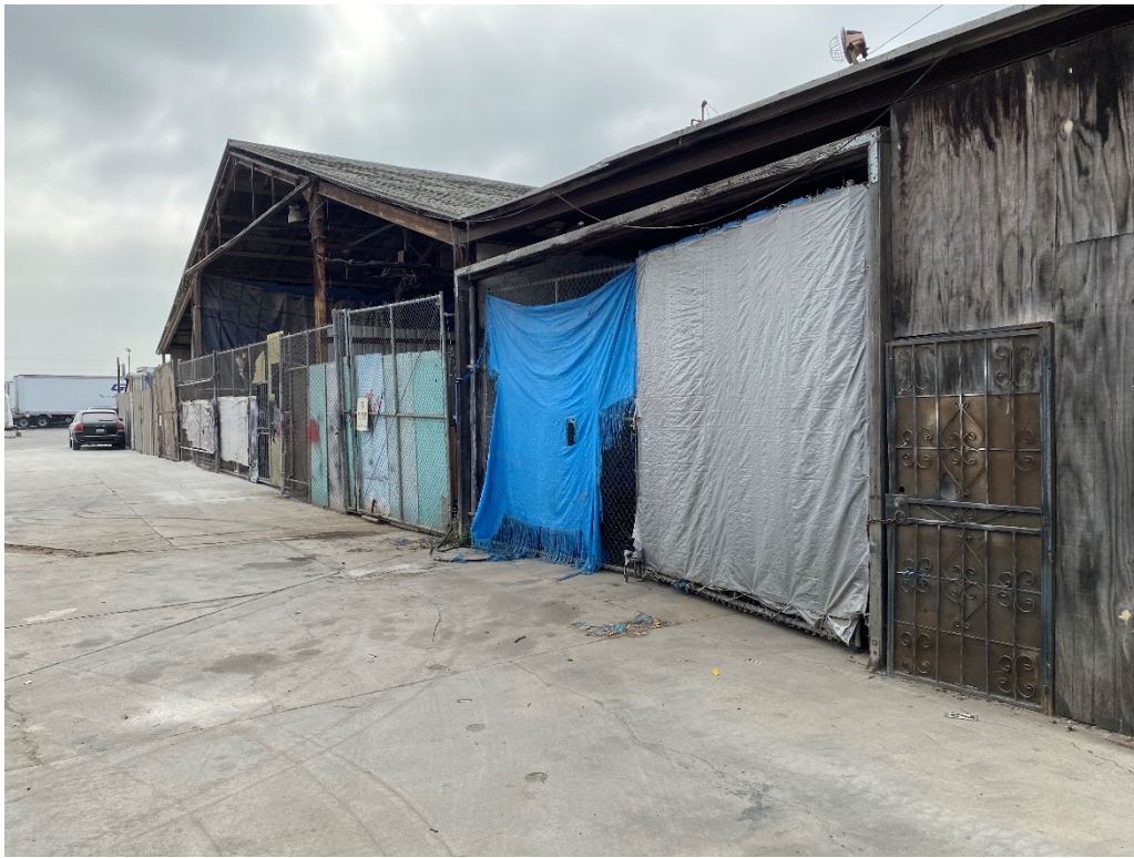
G-5. View of various buildings located at the back of the property (9/3/2021).
