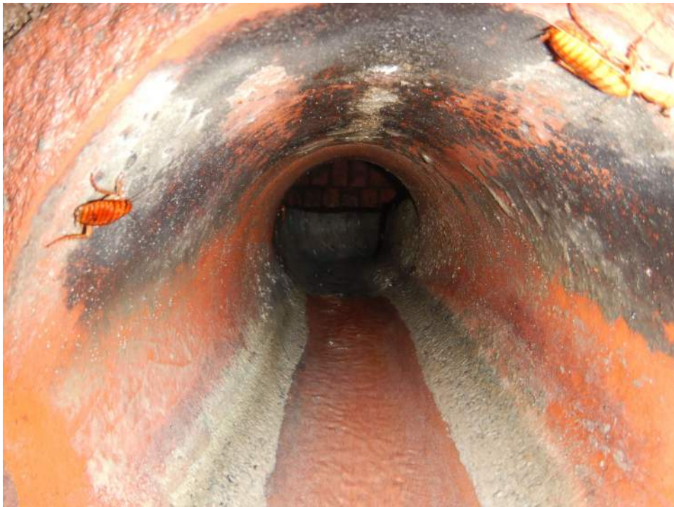
East Influent Pipe
