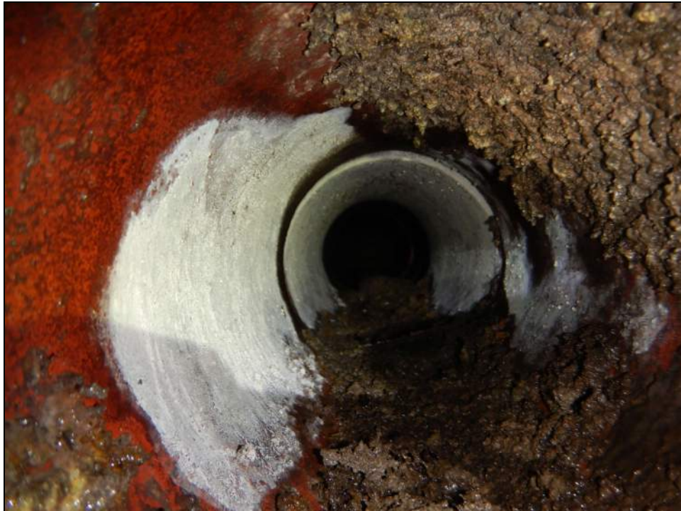
North Influent Pipe, Upper
