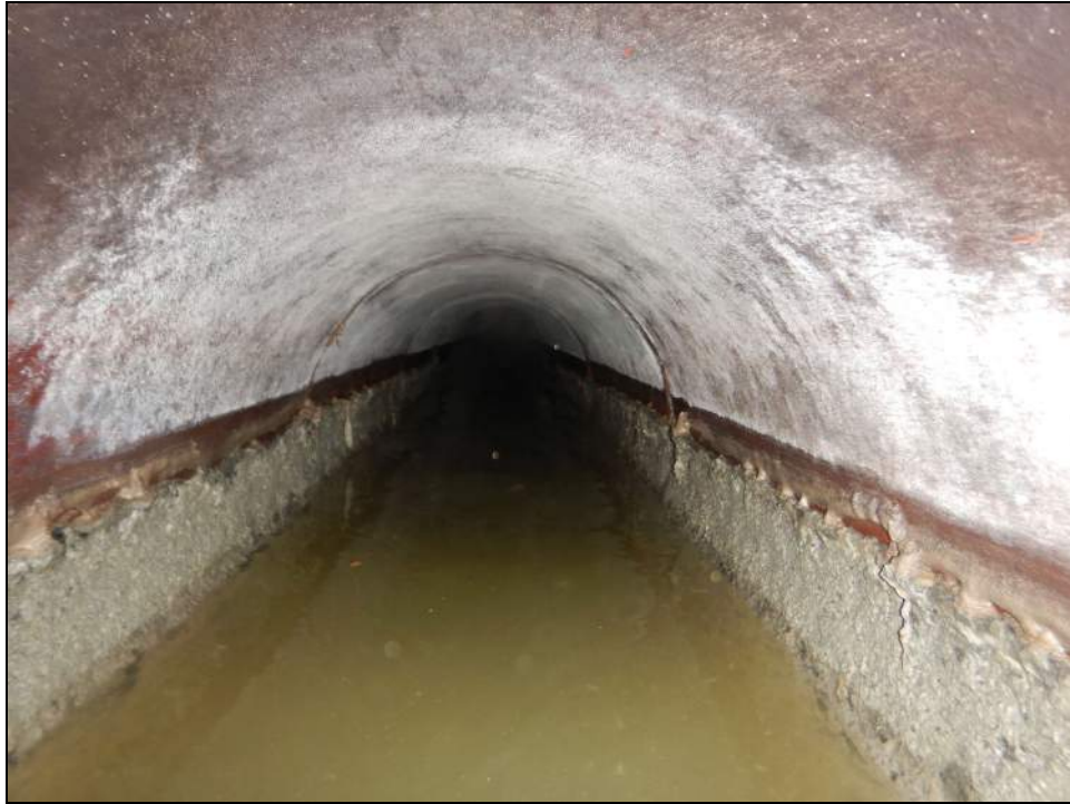
Monitored North Influent Pipe
