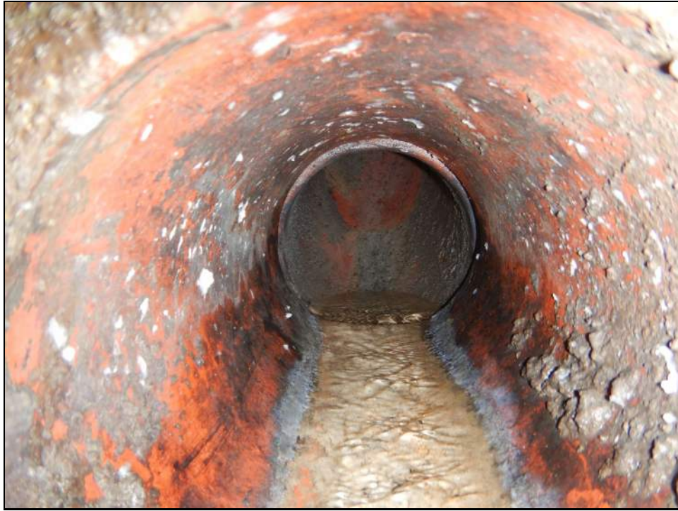
North Influent Pipe, Lower
