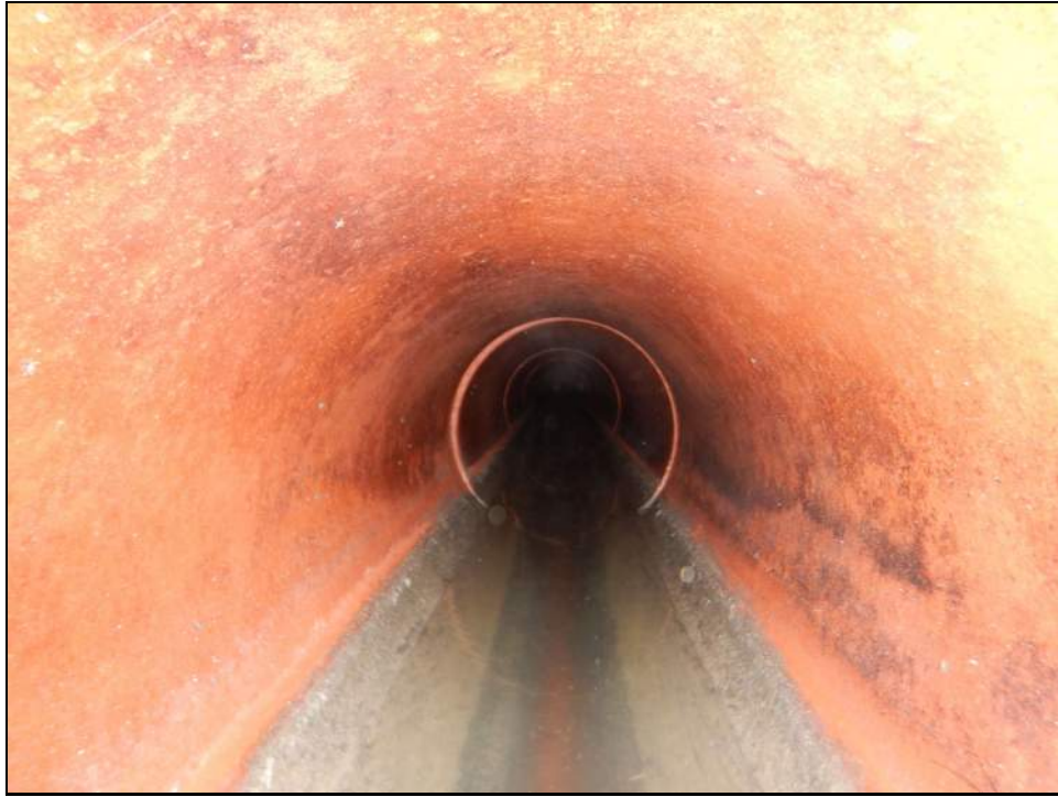
Monitored West Influent Pipe
