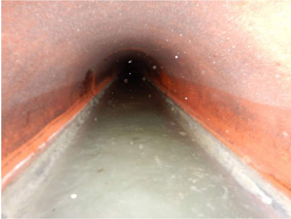
Monitored effluent Pipe
