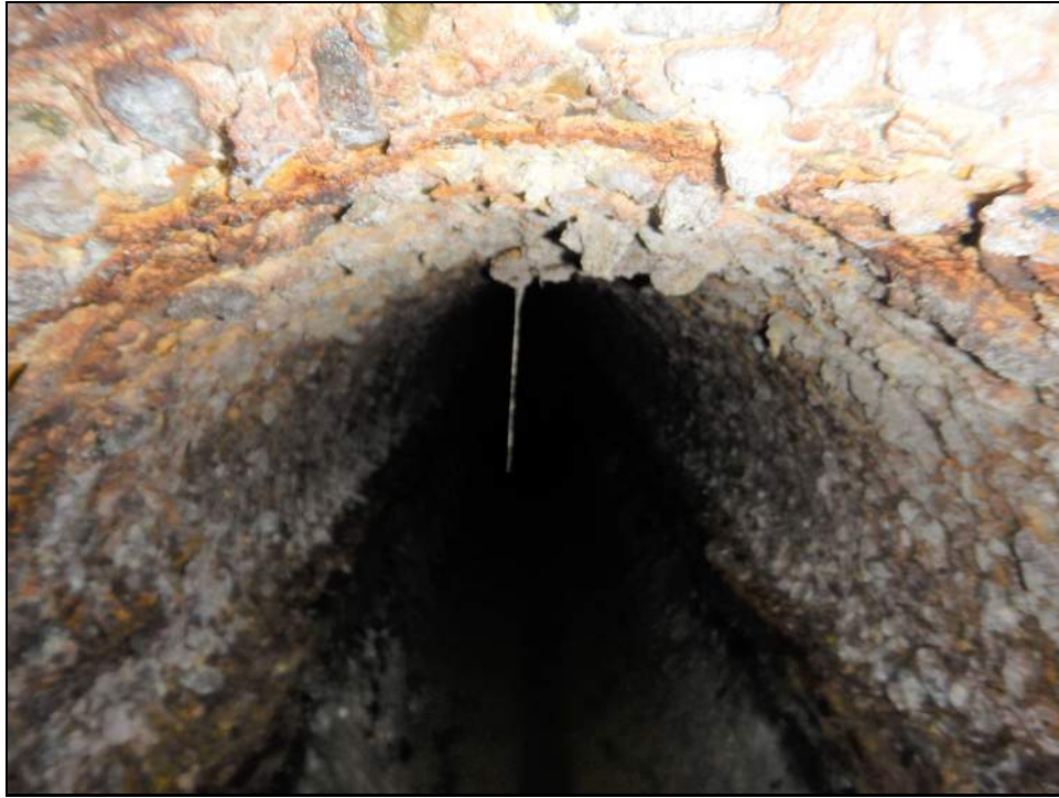
West Influent Pipe
