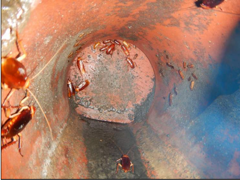
North Influent Pipe
