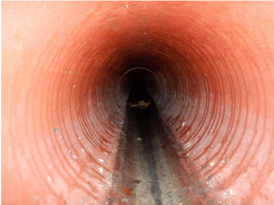
Monitored Influent Pipe
