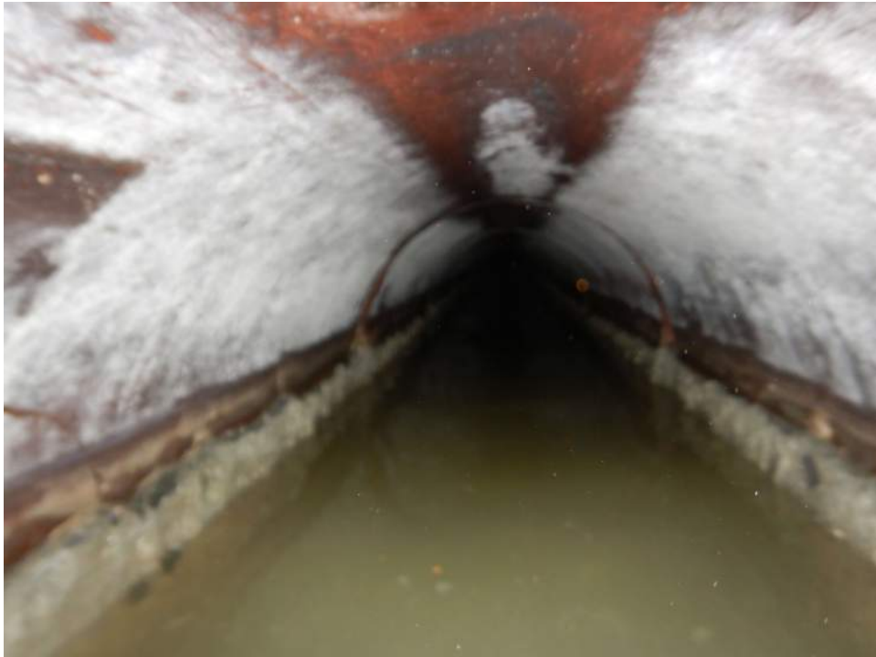
Monitored Influent Pipe
