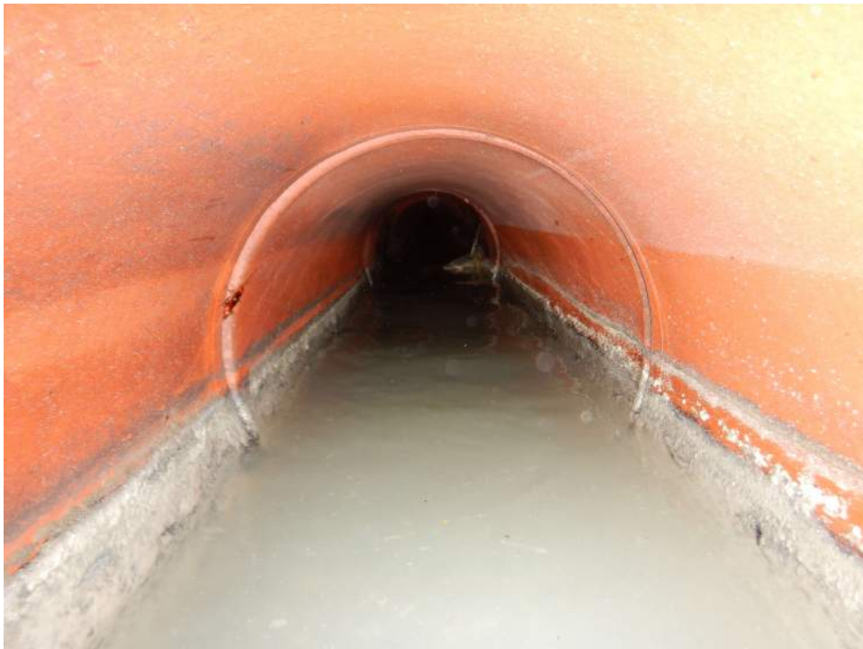
North influent Pipe
