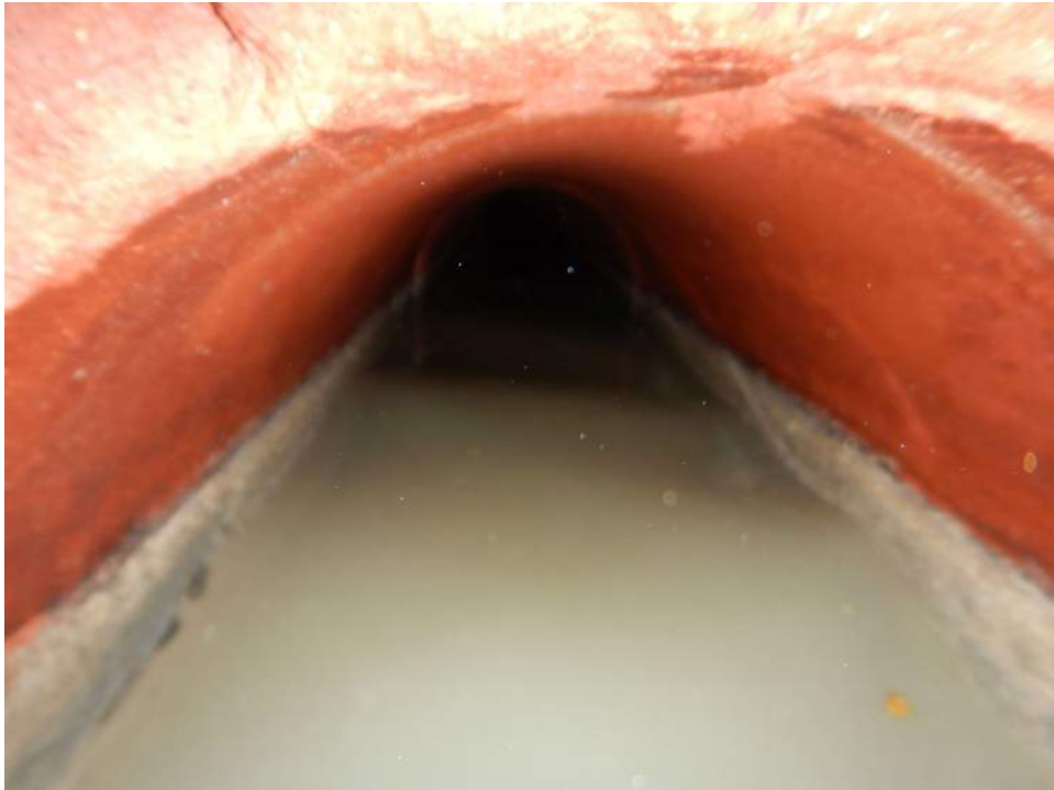
Monitored Influent Pipe
