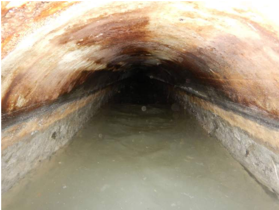
Monitored Influent Pipe
