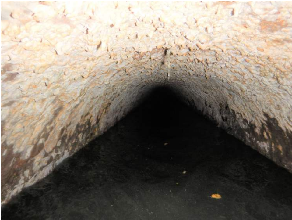
Monitored Influent Pipe
