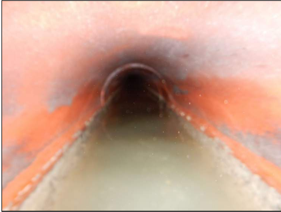
West Influent Pipe
