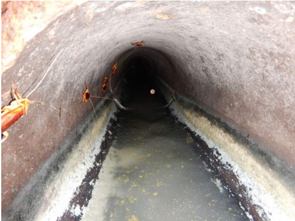
Monitored Influent Pipe
