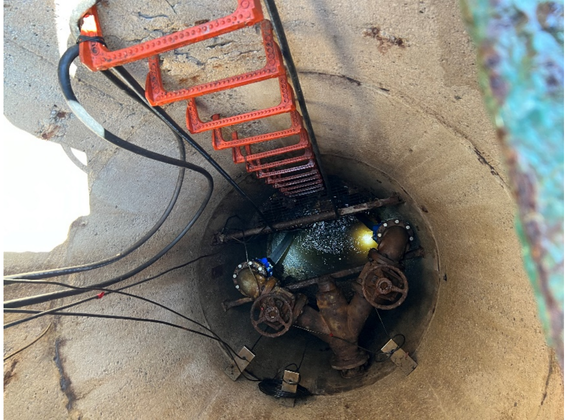
Figure 1.6 Spalling Concrete Around Ladder Rungs
