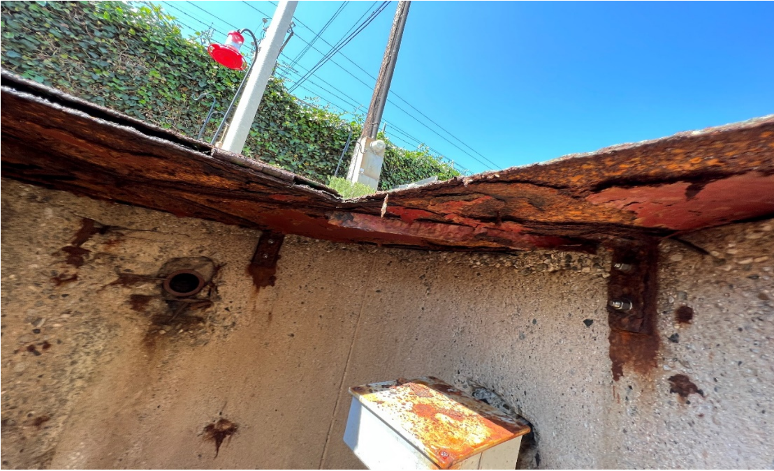
Figure 1.4 Corrosion at Underside of Checkered Steel Plate
