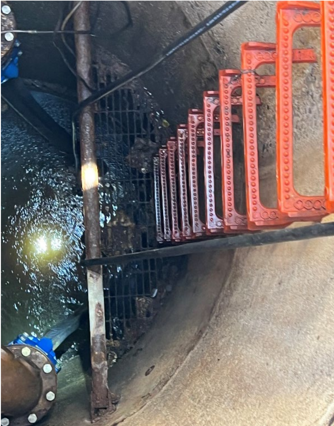
Figure 1.7 Buildup and Signs of Minor Corrosion Around Handrail and Platform Connection to Concrete
