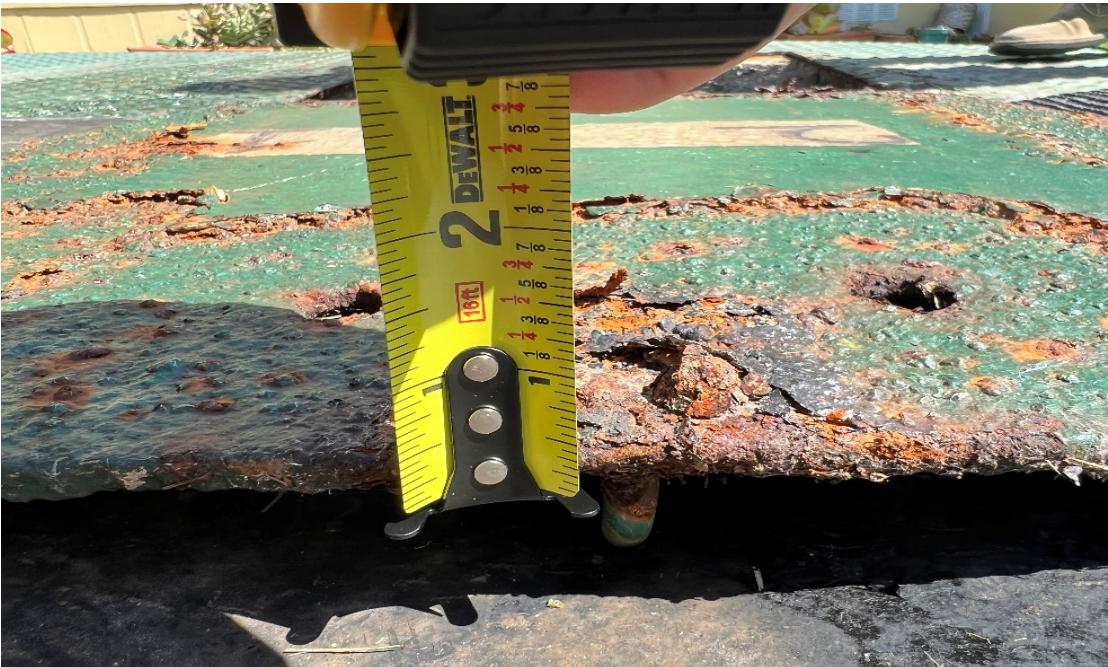
Figure 1.5 Corrosion at Underside of Checkered Steel Plate Hatch
