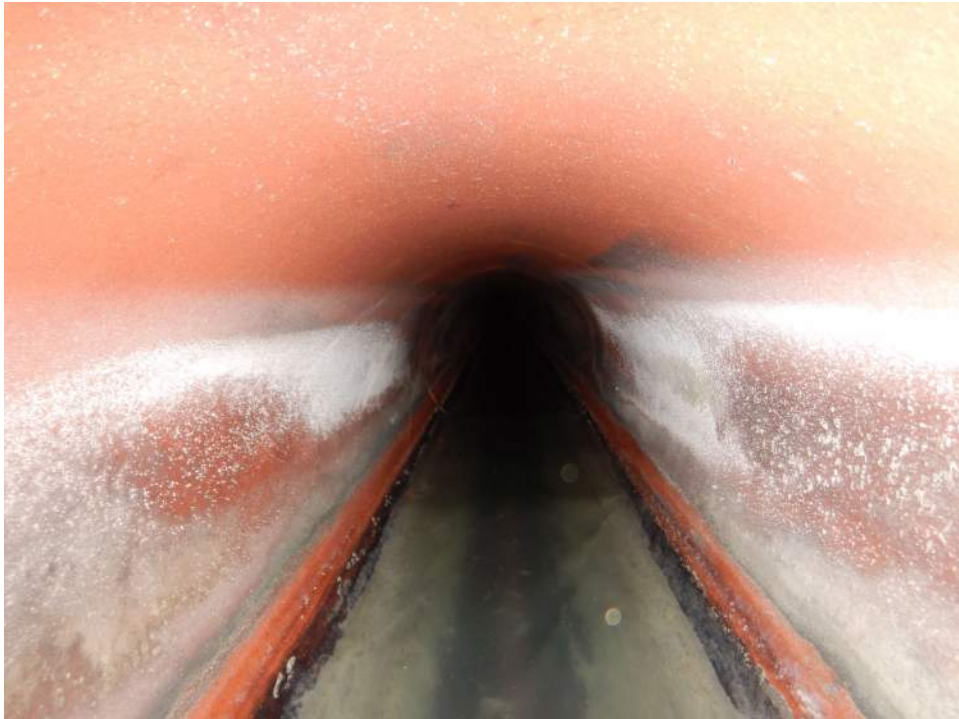
Monitored Influent Pipe
